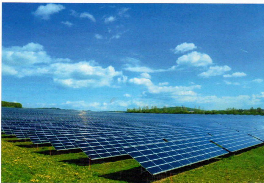
Figure 1: Photovoltaic system on a recultivated landfill field
